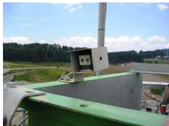
Ultrasonic sensor in the transfer hopper
