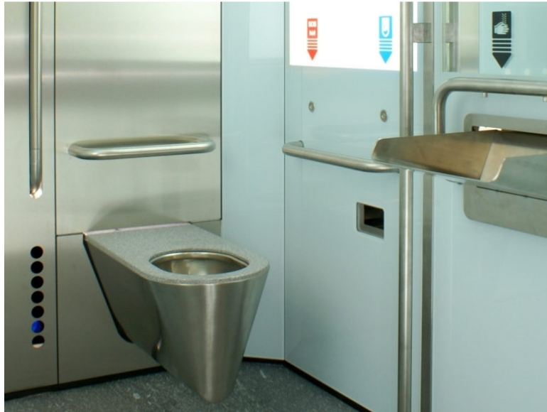
Toilet bowl (cleaning unit behind the stainless wall)
