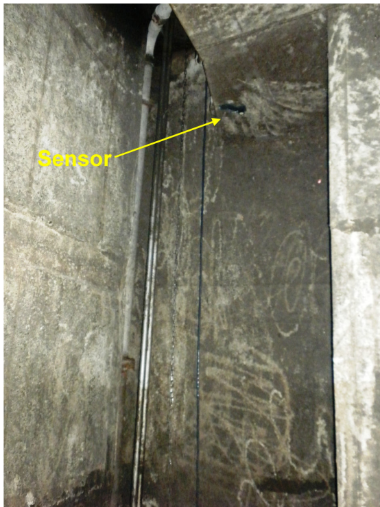
UPK 5000 sensor on the cavern ceiling
